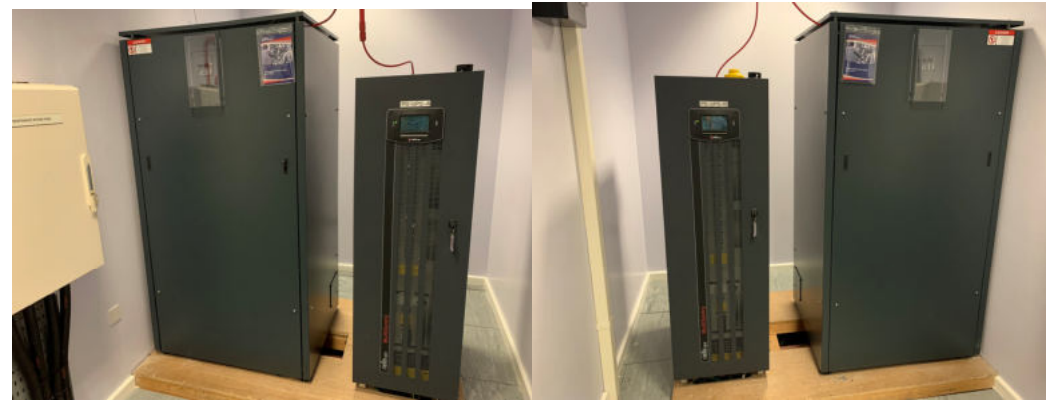
South Block UPS
