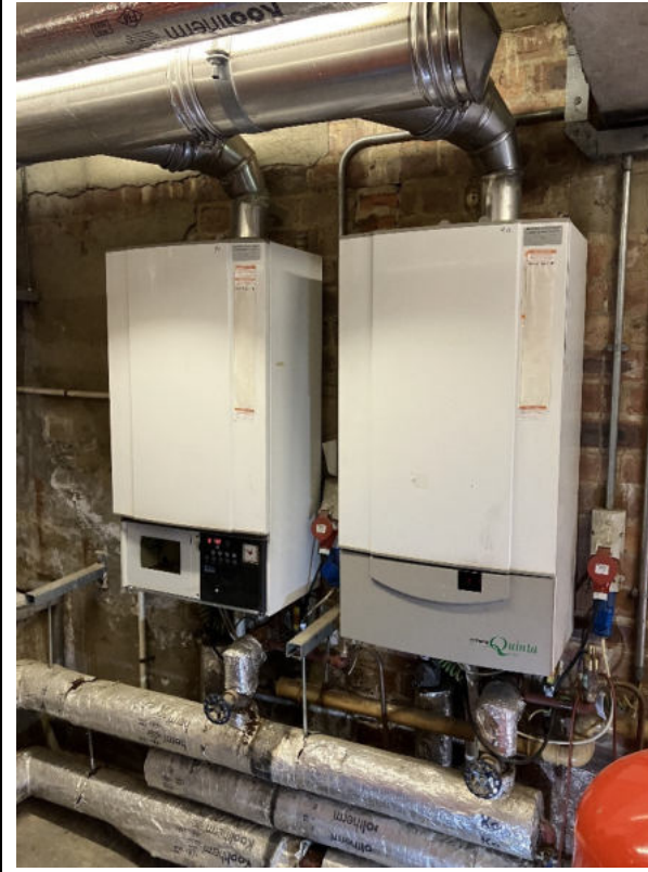
South Block - Boilers
