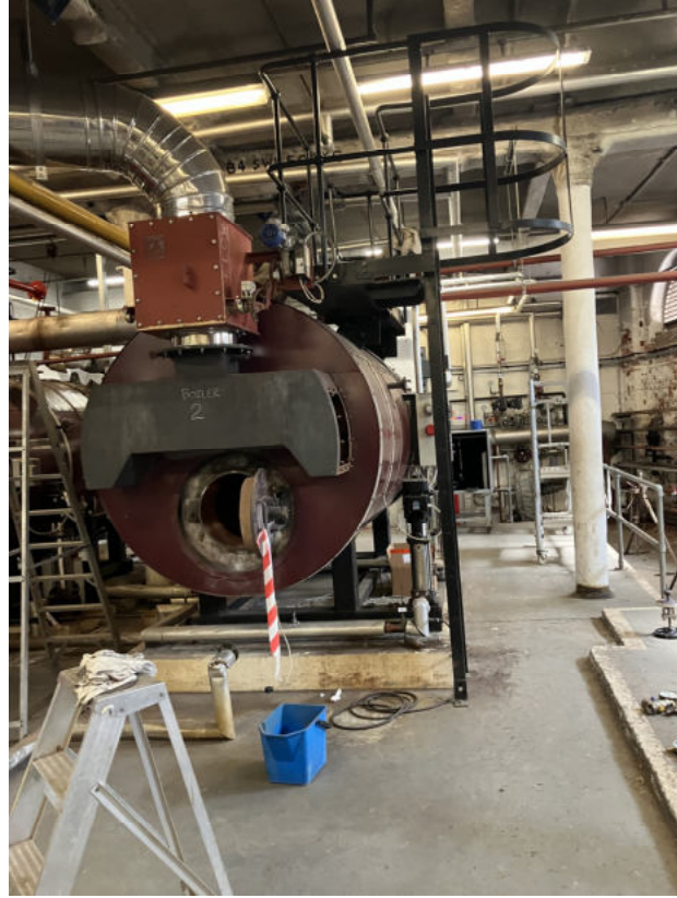
South Block Boiler House – Large Boiler
