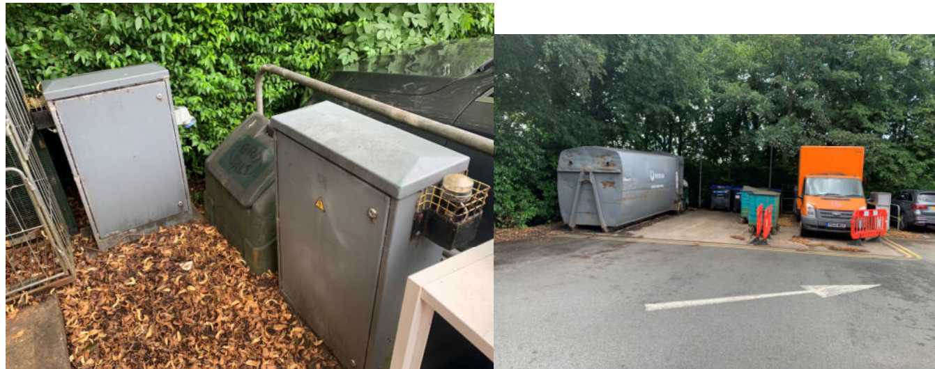
External Feeder Pillar – Entrance to car park
